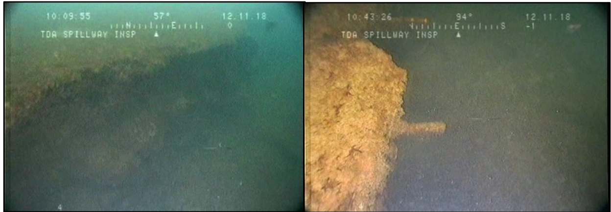
Figure 6 Images showing typical downstream apron end sill erosion along the entire apron downstream of Spillbays 1-8.
